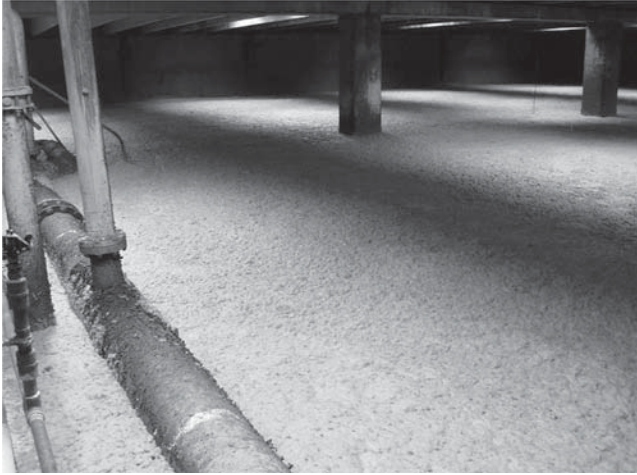
Figure 5.7. Activated sludge basin foaming (approximately 1.5-ft foam) after a chlorine overdose for filament control.
