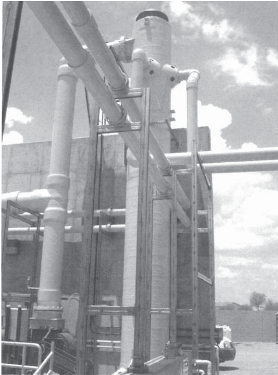
Figure 10.9. Standpipe installation (courtesy of Black & Veatch).
