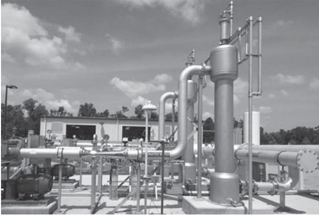
Figure 15.22. Degas separation column (courtesy of Mazzei Injector Corporation).
