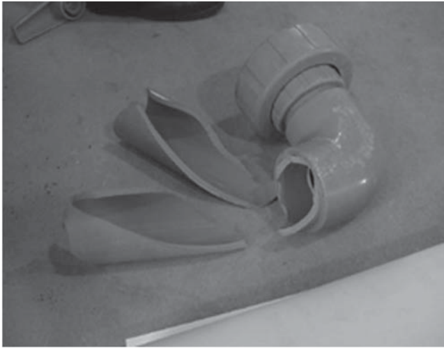
Figure 9.2. Pipe fragments from sodium hypochlorite decomposition without pressure relief.
