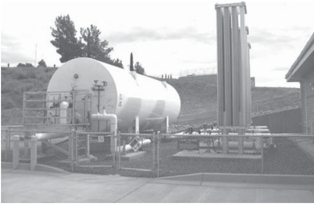
Figure 15.9. LOX storage tank and ambient LOX vaporizer.
