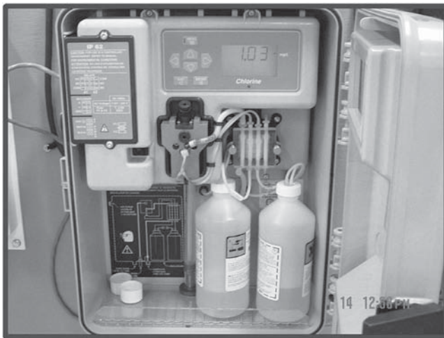
Figure 12.10. The Hach CL17 online chlorine analyzer.
