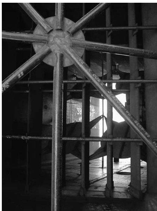
FIGURE 17.20 Static mixers inside the flue gas duct work. (With permission from Haldor-Topsoe, Inc.)
