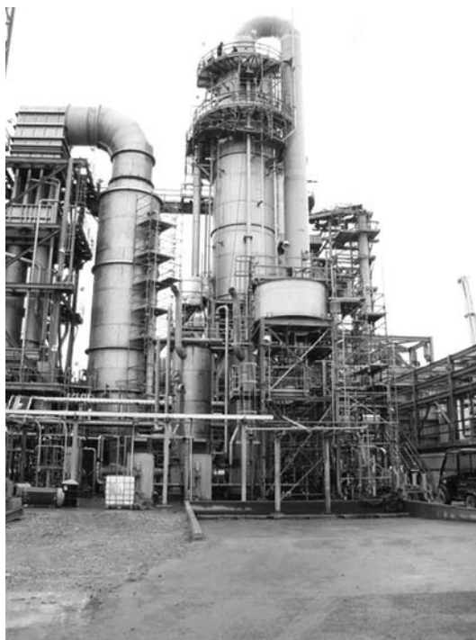
FIGURE 17.29 Commercial LoTO x unit layout at Marathon's Texas City Refinery. (With permission from Belco Technologies.)
