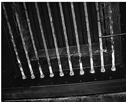
FIGURE 17.11 ABS corrosion on \text{NH}_3 injection lances. (With permission from Haldor-Topsoe, Inc.)
