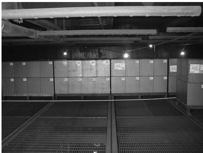
FIGURE 17.18 Catalyst modules loaded inside SCR reactor. (With permission from Haldor-Topsoe, Inc.)
