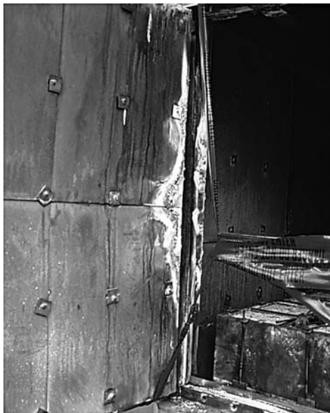
FIGURE 17.10 ABS corrosion on SCR access door. (With permission from Haldor-Topsoe, Inc.)
