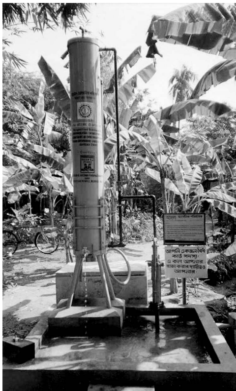
Figure 2 Wellhead arsenic removal unit. (See insert for color representation of figure.)
