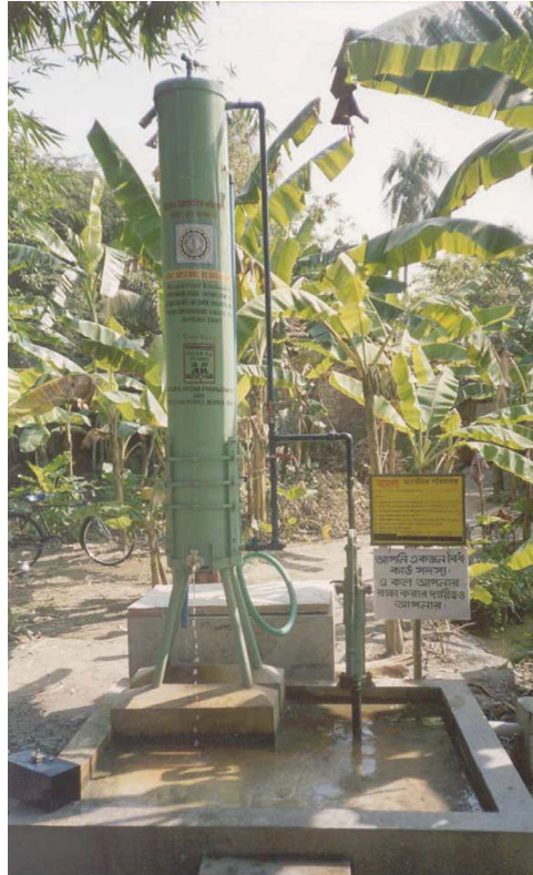
Chapter 13, Figure 2 Wellhead arsenic removal unit.
