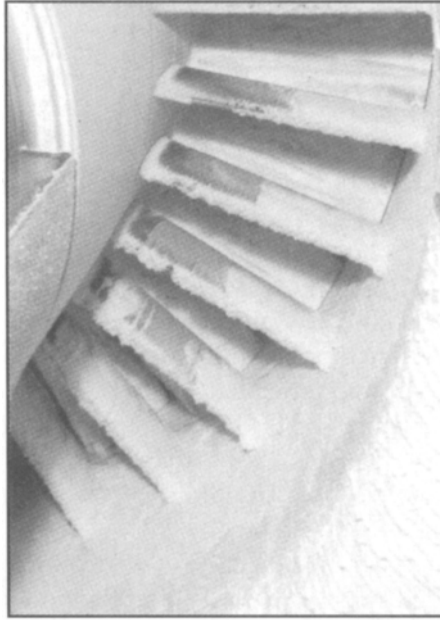
Figure 4-27. Ammonium nitrate salt deposits in the inlet of a nitrous gas axial compressor.
